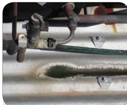
Figure 1 Bi-metallic corrosion caused by "copper-rich" water run-off
