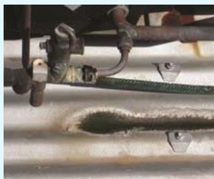
Figure 1: Bi-metallic corrosion caused by ‘copper-rich’ water run-off
