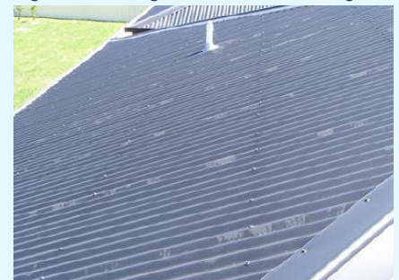
Figure 2: Roofing with sunscreen damage
