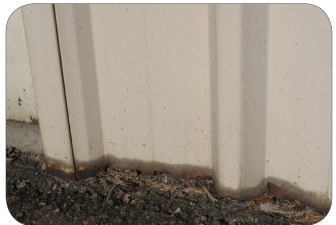
Figure 2: Corrosion due to inappropriate wall design
