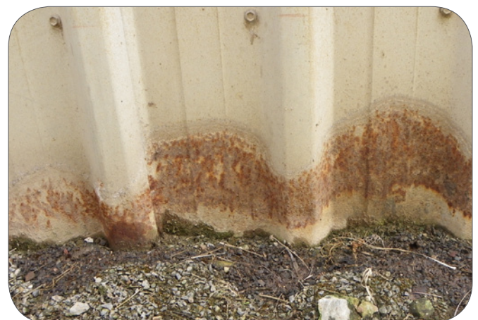
Figure 3: Corrosion due to soil immersion
