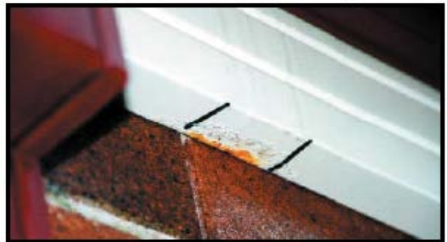
Figure 1: Example of corrosion caused by incorrect acid brick cleaning practises.
