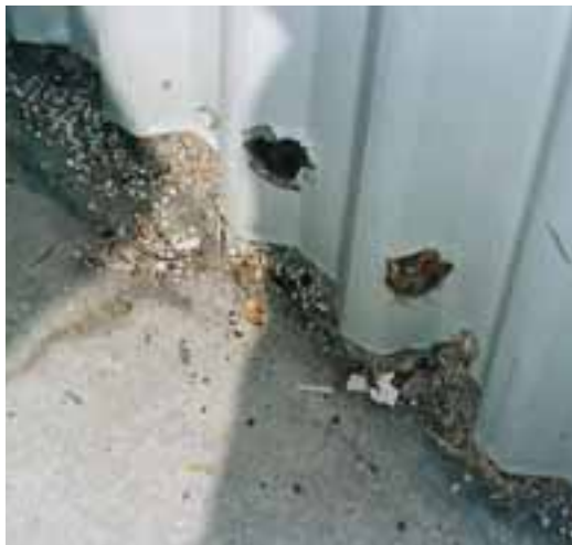
Figure 1: Example of corrosion resulting from contact with fertilizer.
